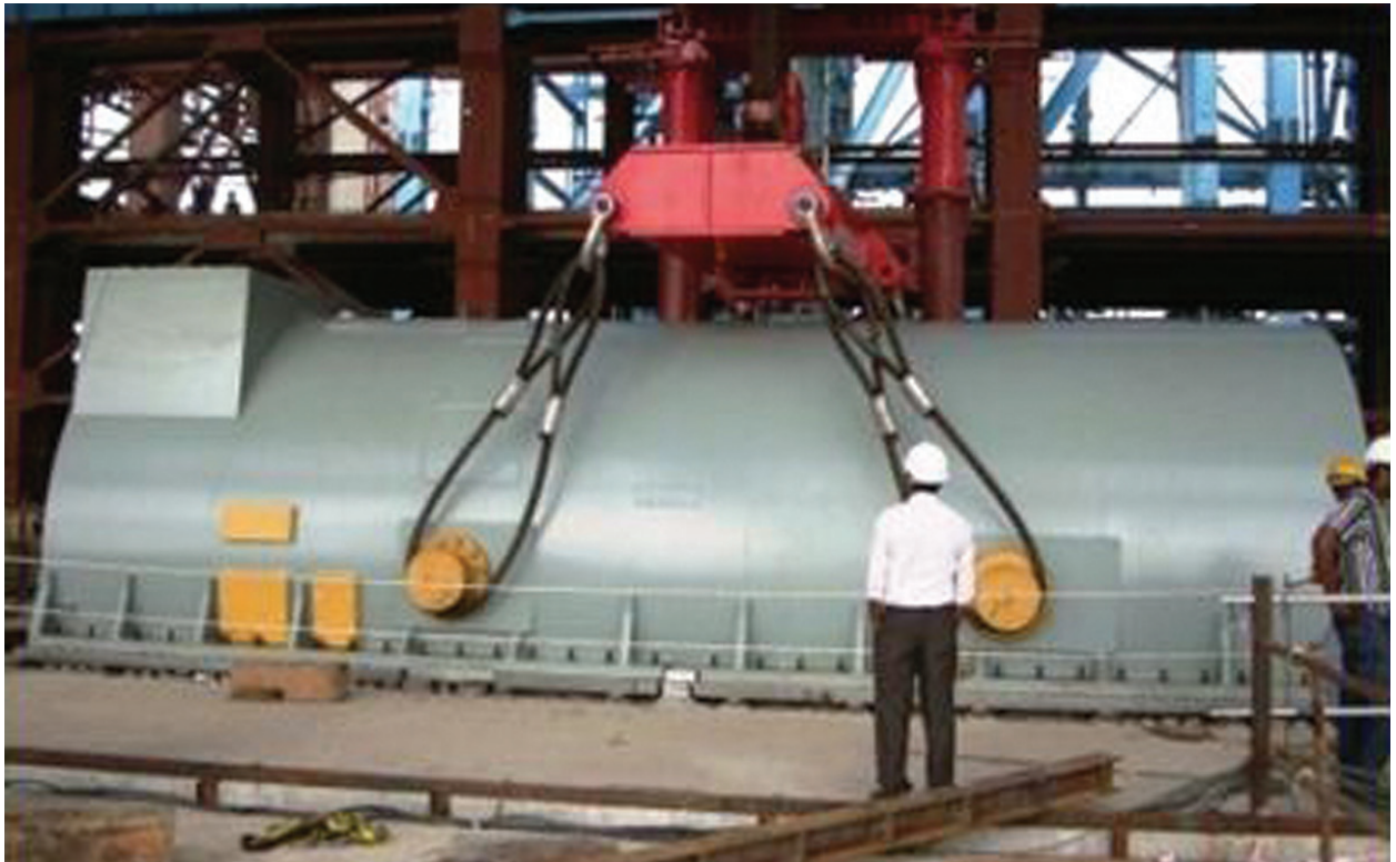
Koradi Generator Stator
